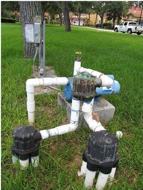
Three indexing valves... want to guess which zone is irrigating?
